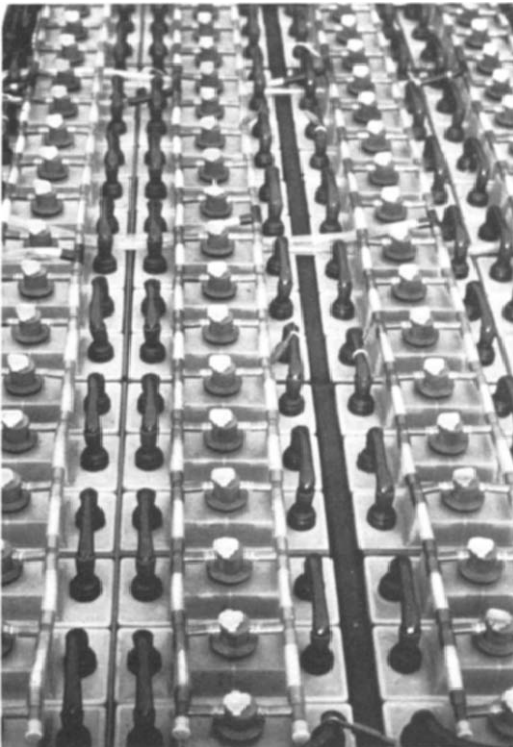
Fig. 8. Battery with water refill system and central degassing.
